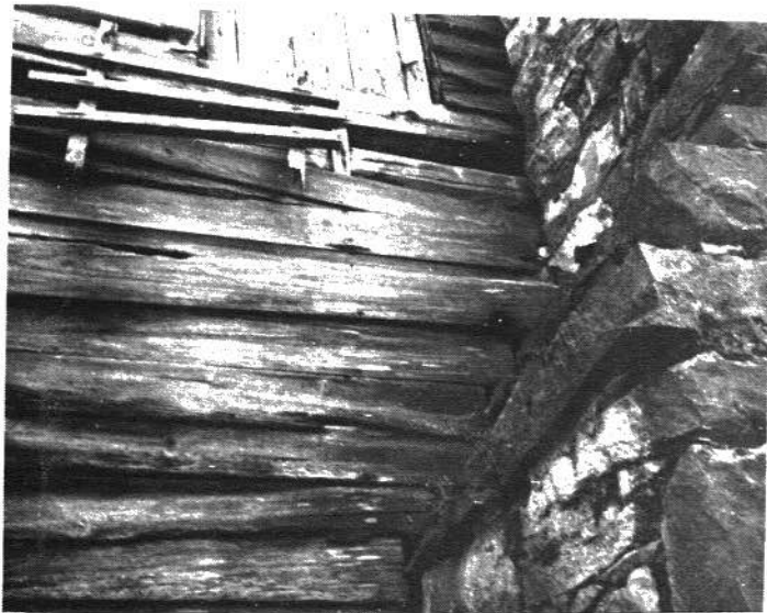
Here you can see the logs under the window by the chimney. The shutter in the window will swing in and out. Also, notice what is left of the ladder under the window.
